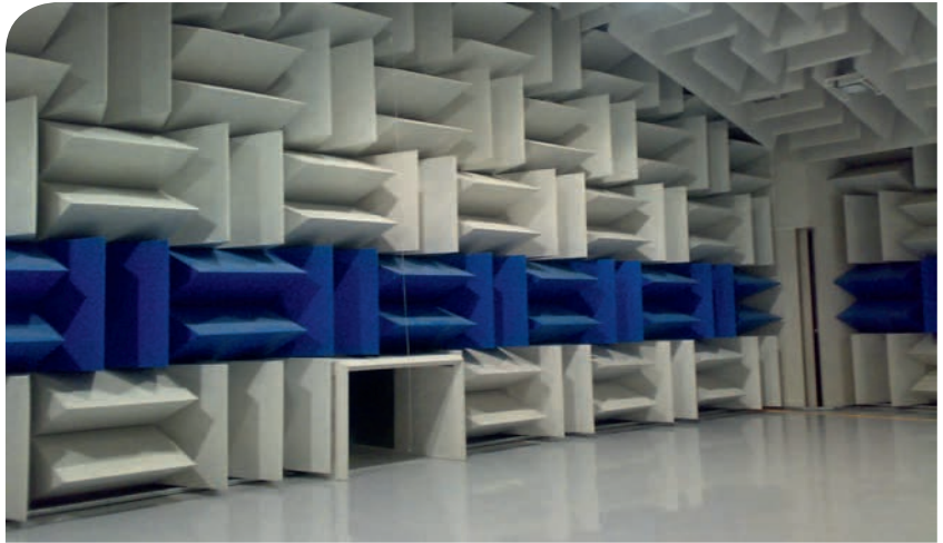
Typical forced air cooling duct system in vehicle hemi-anechoic Chamber
