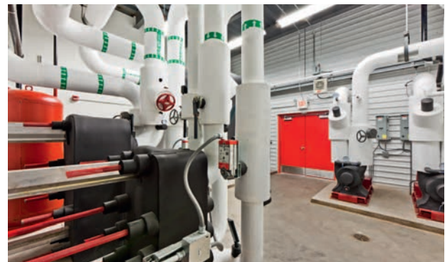
Plant room for turnkey acoustic testing facility
