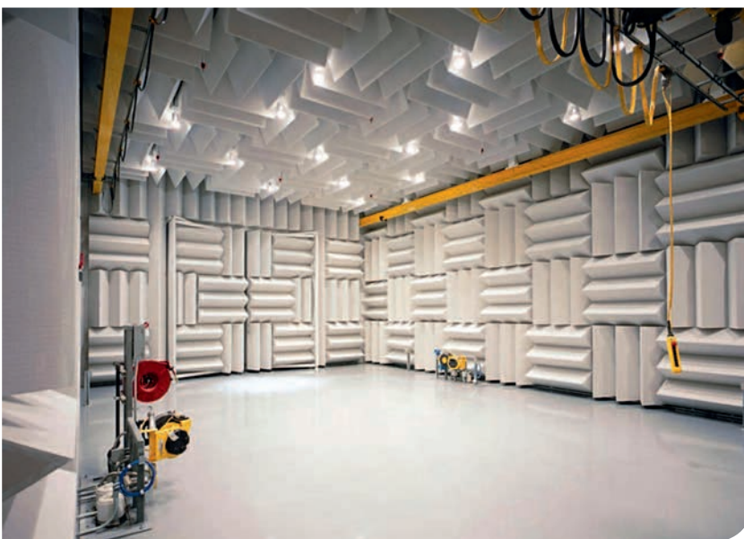
A typical IAC quiet room facility
